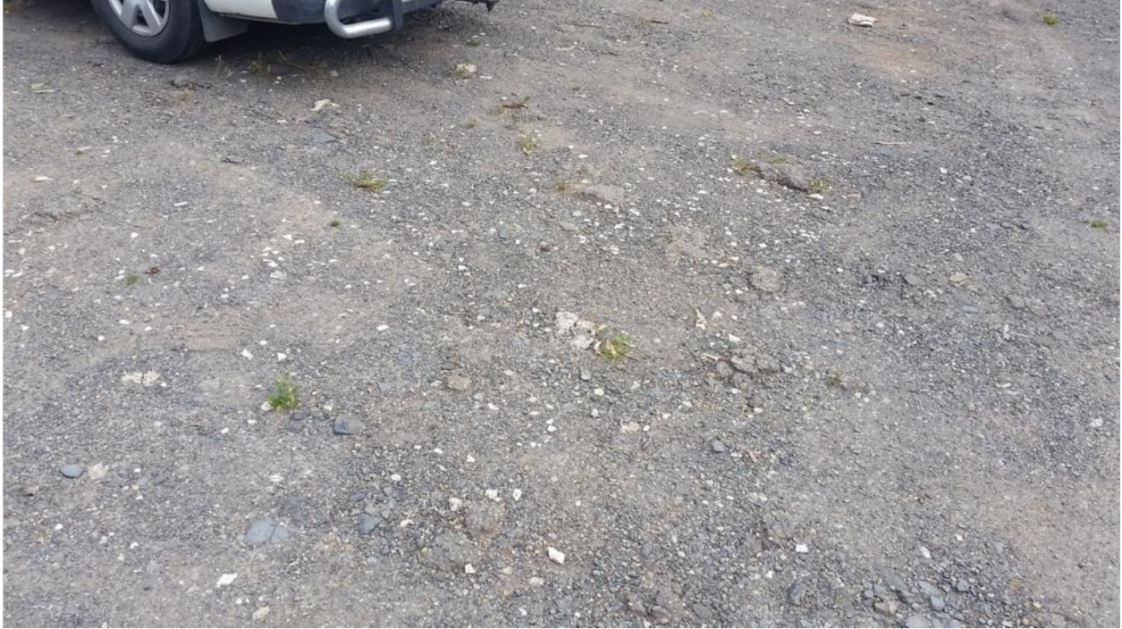
Photo 7: Crushed asbestos- sheeting fragments located within the gravelled car-park in the southern portion of the site.
